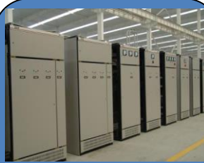
低压进、出线柜
